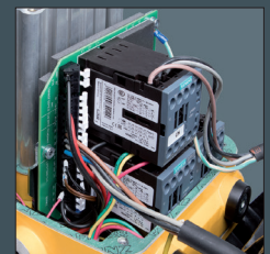
LOW VOLTAGE CONTROL
